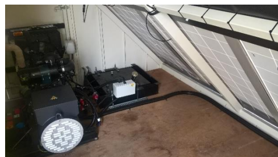
Figure 07 – Interior of Solatainer
