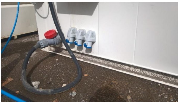
Figure 06 – Electrical plug points on the side of Solatainer
